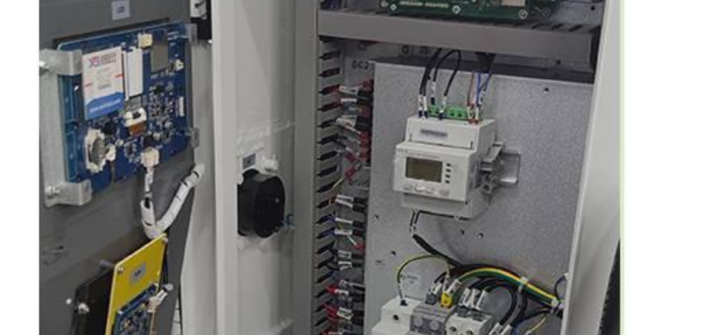
Wiring with Shunt
